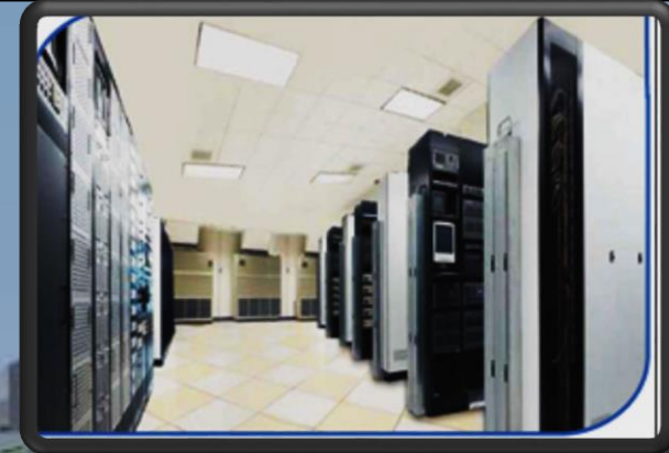
Energy Efficient Data Center
