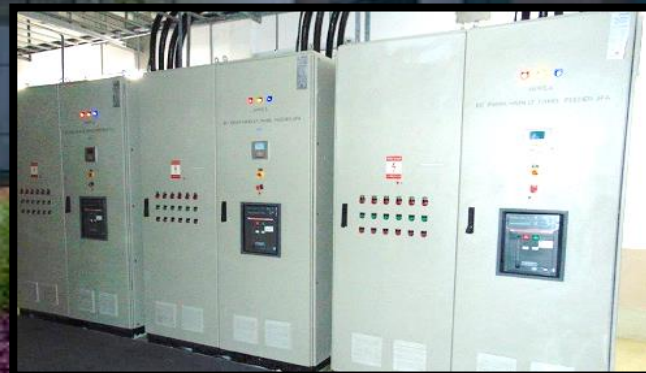
Automatic Power Factor Control
